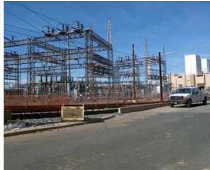
a BGE substation
