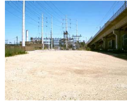
a BGE substation
